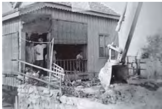
A house of affectees who refused to relocate for the HW1 project. They are being intimidated with a bulldozer. (Source: The NGO Forum on Cambodia, 2000)
