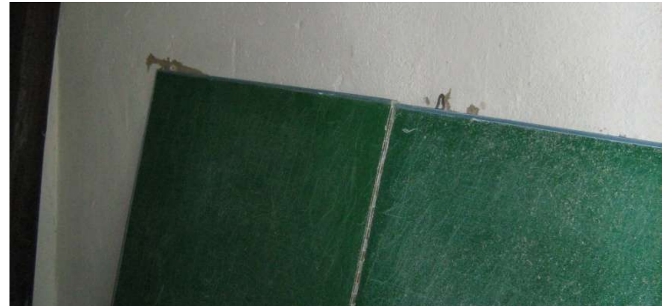
The newly installed blackboard in one of the classrooms was already broken after days of being used—one of the proofs of the substandard quality of work in the project.
