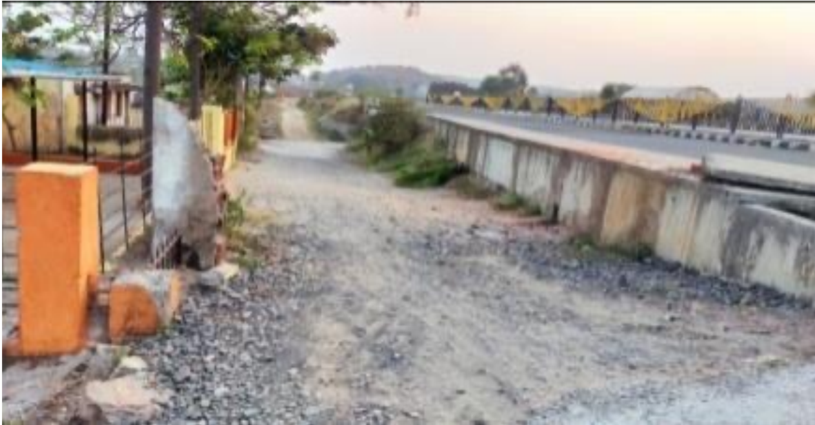
Poorly constructed service roads
