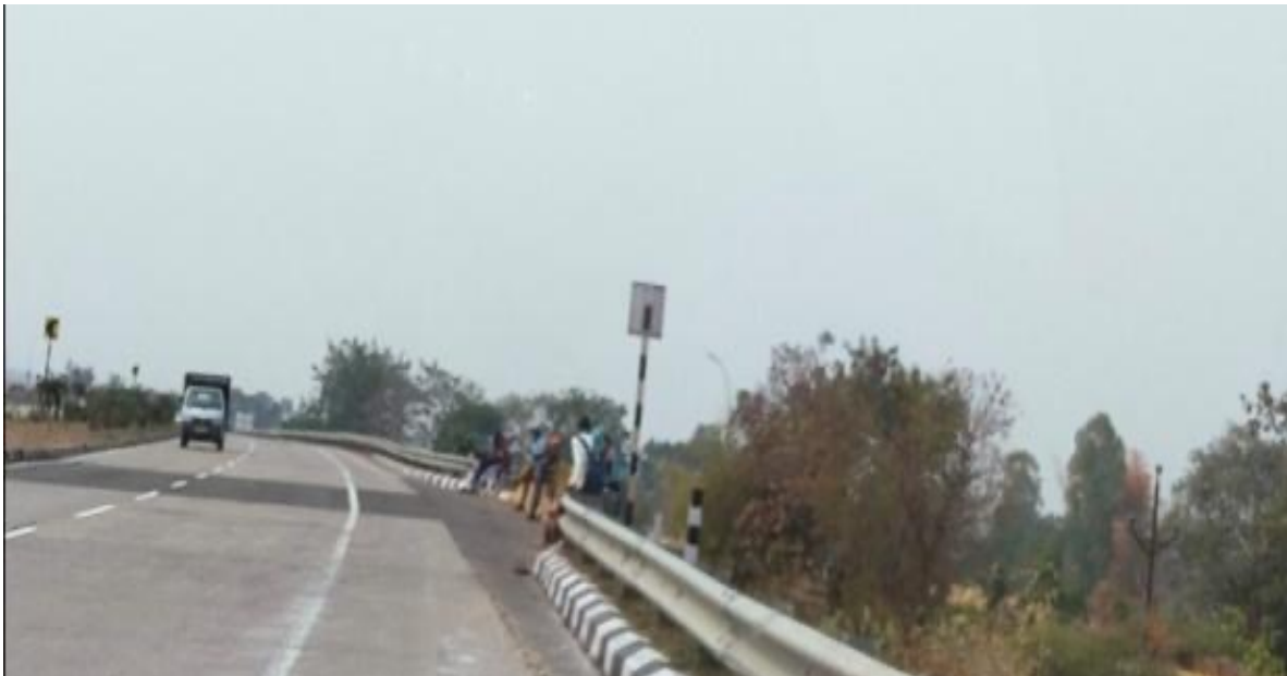
Lack of waiting area, students having to wait on highway (NH-69)
